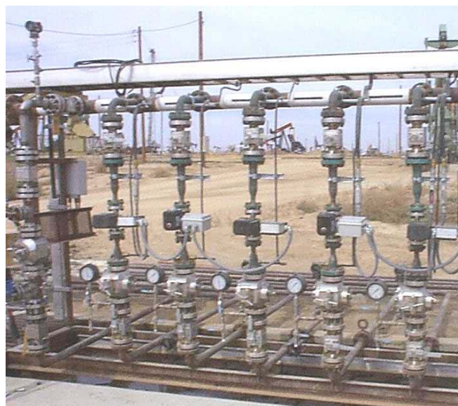
Figure 20. Automated injection header
