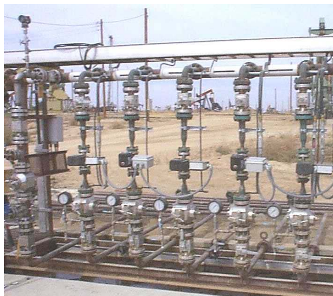
Figure 20. Automated injection header
